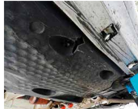
Damage to the underbody panelling
